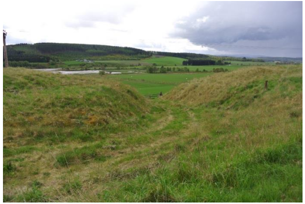
Disused rail line, missing bridge
